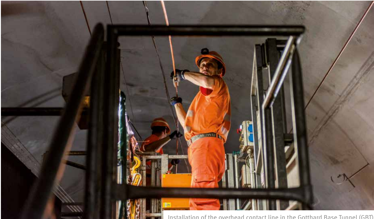
Installation of the overhead contact line in the Gotthard Base Tunnel (GBT)
