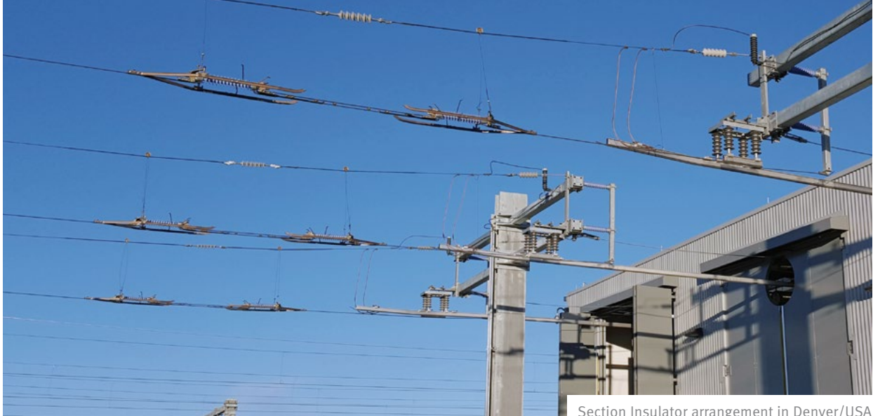
Section Insulator arrangement in Denver/USA
