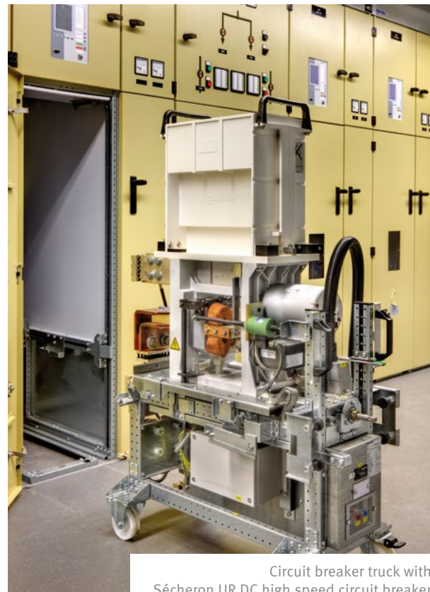
Circuit breaker truck with GE Gerapid DC high speed circuit breaker
