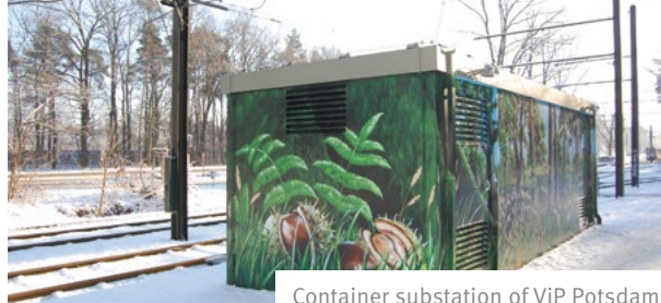
Container substation of ViP Potsdam
