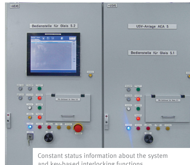
Safely working on the vehicle roof: TracFeed® AEA ensures that the catenary is shutdown and earthed before the work is started
