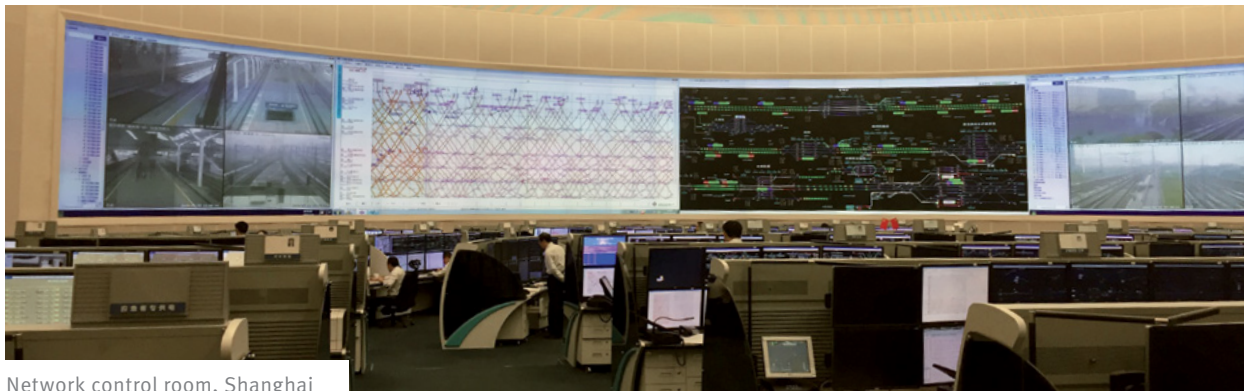
Network control room, Shanghai
